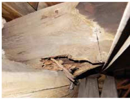
View of crushed and decayed timber.
