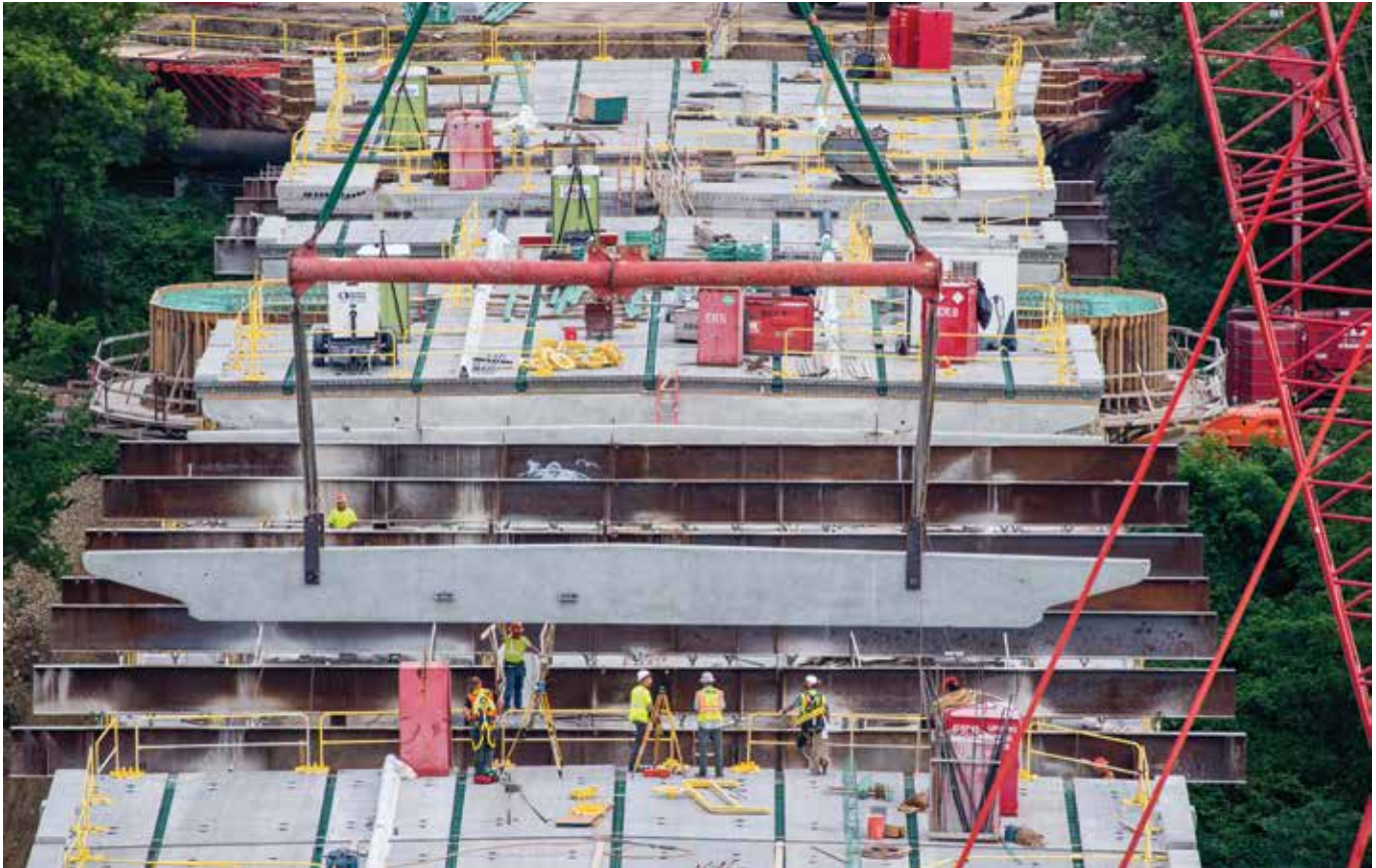
Fig. 8: An overview of the ABC process. In the foreground, a new cap beam is being placed. New deck panels are already in place in adjacent spans (photo courtesy of HNTB Corporation and Joe Szurszewski Photography LLC)
