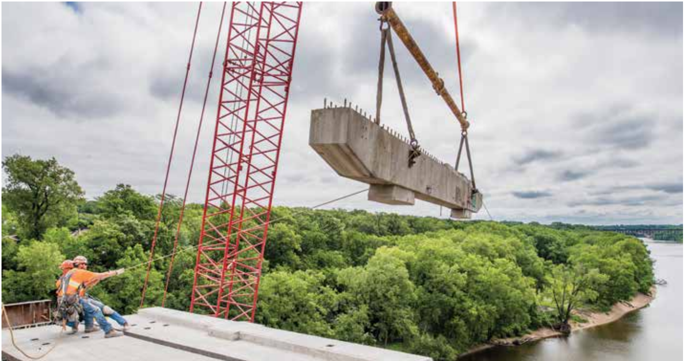
Fig. 7: Workers remove an existing cap beam from the structure (photo courtesy of HNTB Corporation and Joe Szurszewski Photography LLC)
