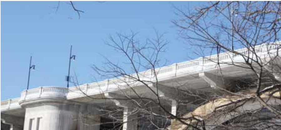
Fig. 6: Ornamental railings were constructed using architectural precast concrete (photo courtesy of Koichiro Shimomura)
