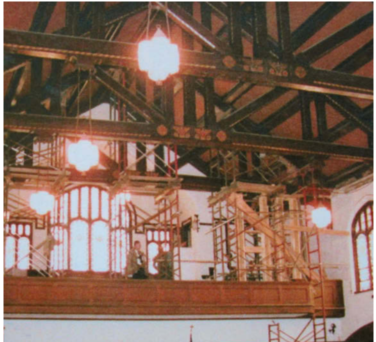
Partial view of church sanctuary with temporary shoring in place at failed truss. Closer view of truss end reconstruction in progress with new preservative treated glulam.
