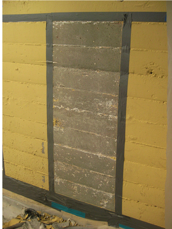
The exposed concrete surface and form board pattern and texture were part of the original character of the facade of this historic concrete structure. Trials were conducted to evaluate removal of the coating that had been applied later in the life of the building.
