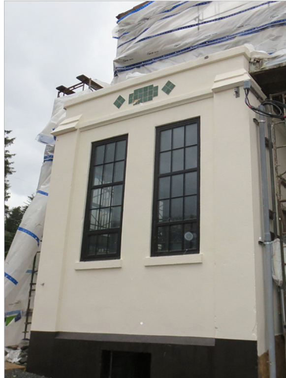
This early twentieth-century historic concrete building had originally been coated; the existing deteriorated coating was removed and a new coating system applied to match the historic appearance.
