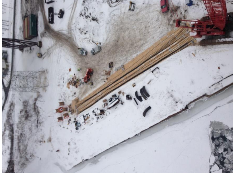
Figure 12: Counterweight ropes pulled off the shipping reel in preparation for installation with a crane.
