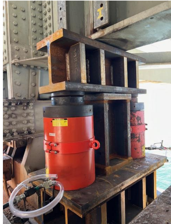
Figure 4: Jacking assembly located under lift span end floorbeam. The assembly included an added local dump line (clear tubing) to facilitate retracting the cylinders.
