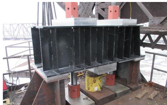
Figure 5: Counterweight jacking assembly located at the top of a tower.
