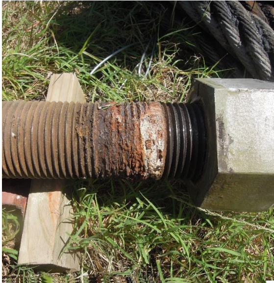
Figure 2: Heavily corroded threads were discovered in the portion of the take-up that passed through the billet.
