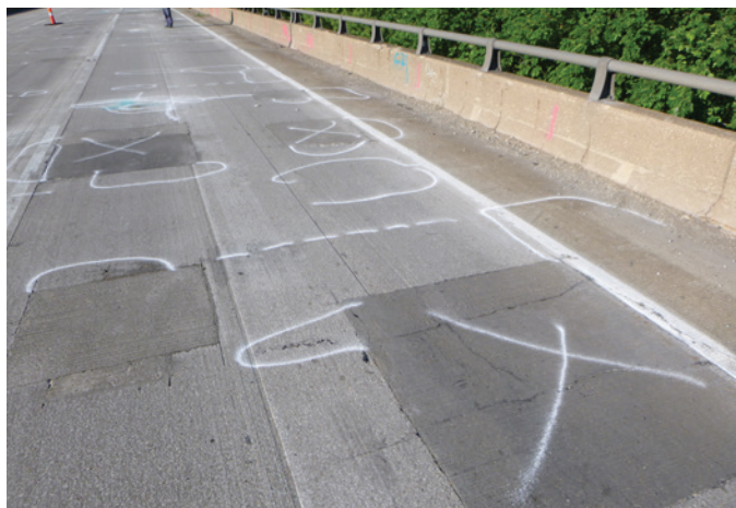
Fig. 4: Example of a bridge deck with previous repairs, cracks, and delaminations identified from visual inspection and conventional chain-drag sounding techniques
