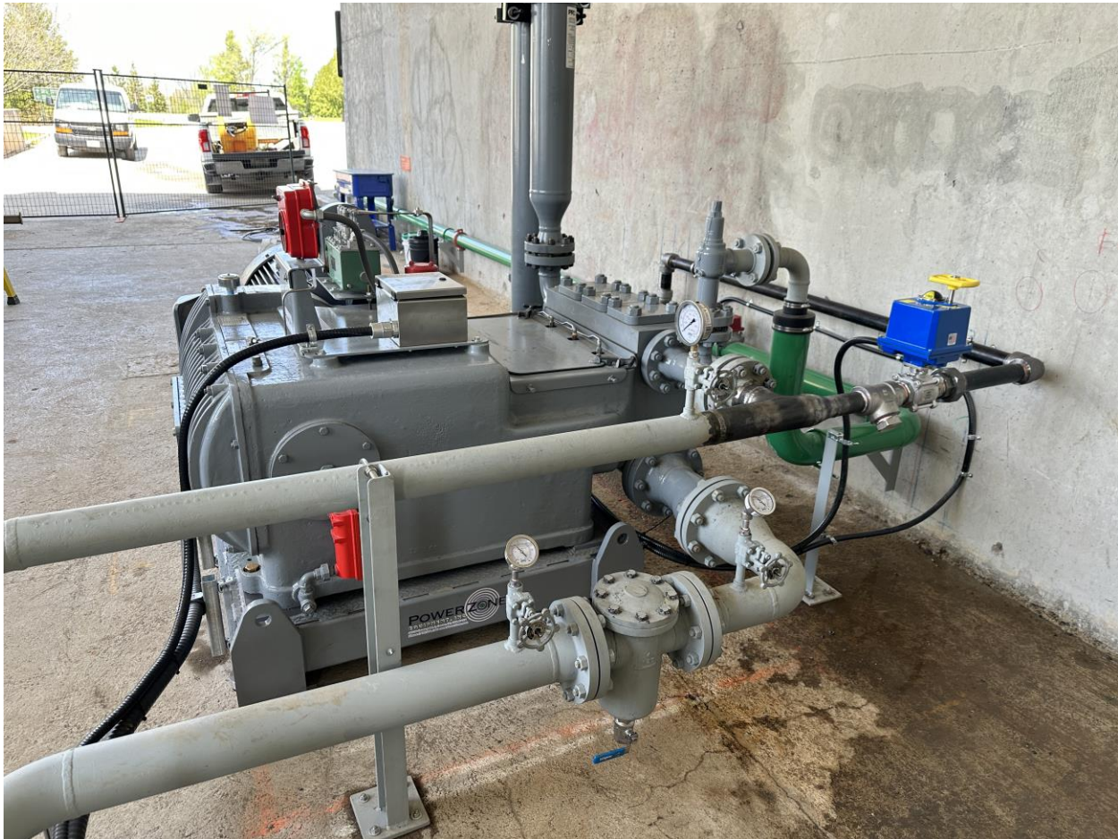
Figure 8 New 150 hp Pump for Single Chamber Operation
