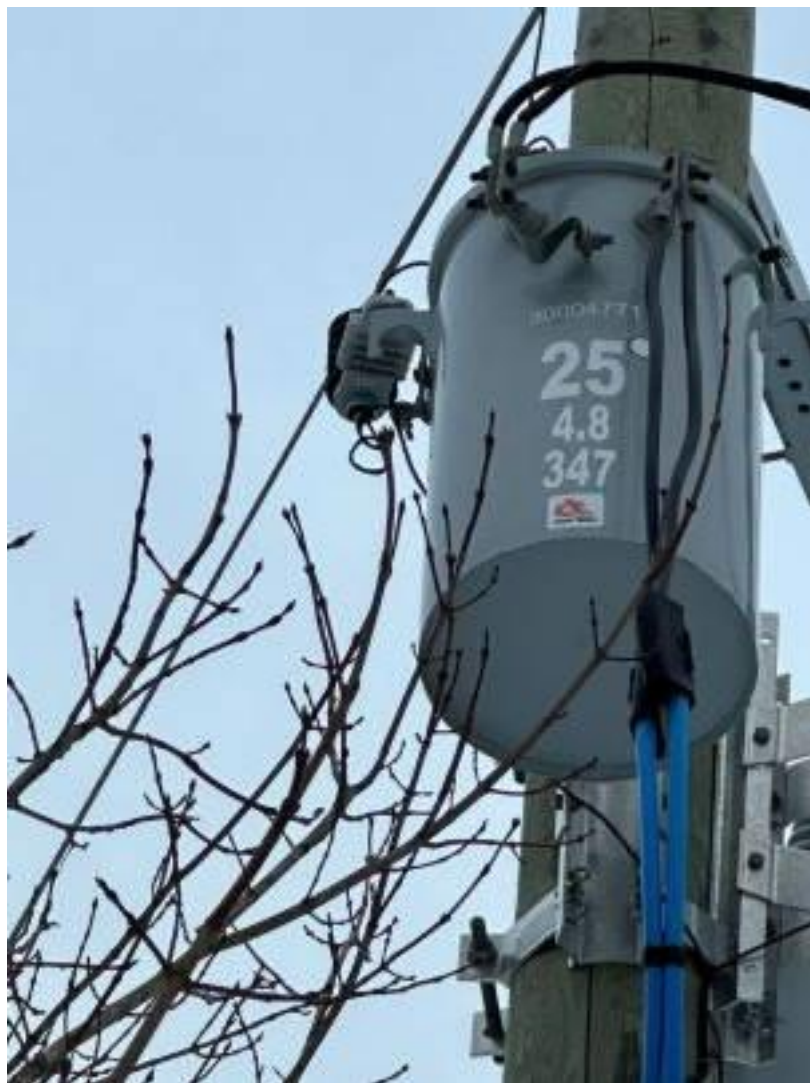
Figure 9 Electric service transformer prior to upgrade which was inadequate to support 150hp operation.
