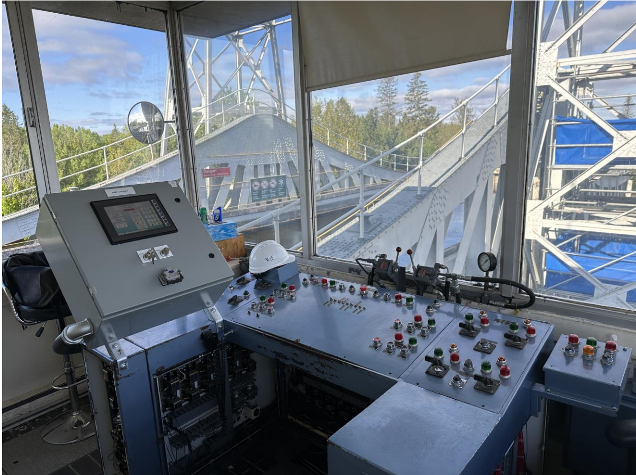
Figure 10 Piggyback control system mounted on existing control desk.
